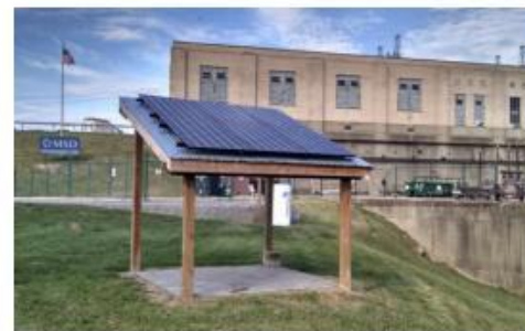
Figure 2. Solar panels for powering the water pump.
