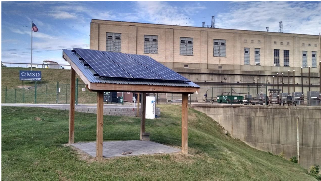
Figure 3.2 Panels for Powering Water Pump
